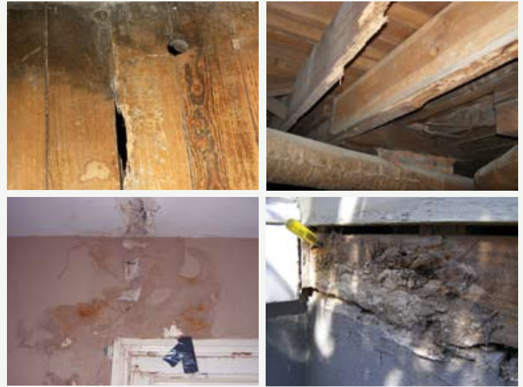
These images of the Woodrow Wilson Home illustrate the degree of damage found throughout the structure.
